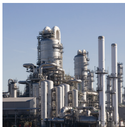
Fractionating towers, reactors and catalyzers
